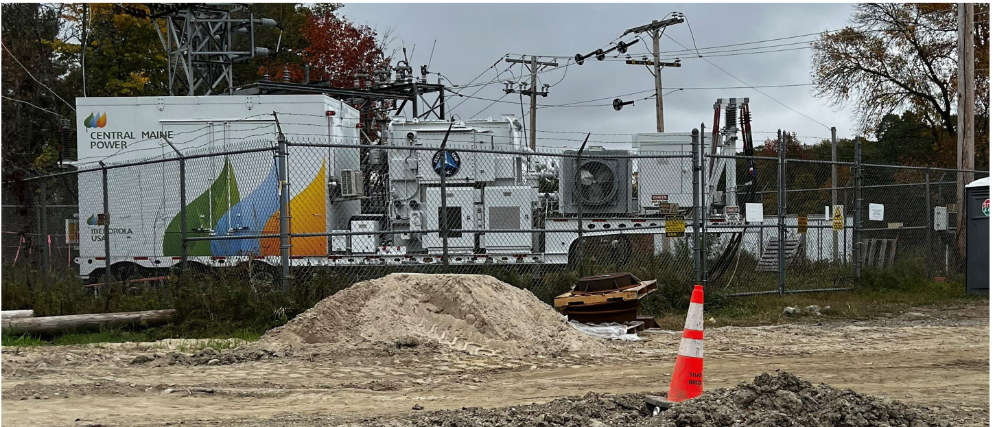
Current Biddeford Pump Substation off South Street in Biddeford, Maine shown with a mobile transformer installed.
