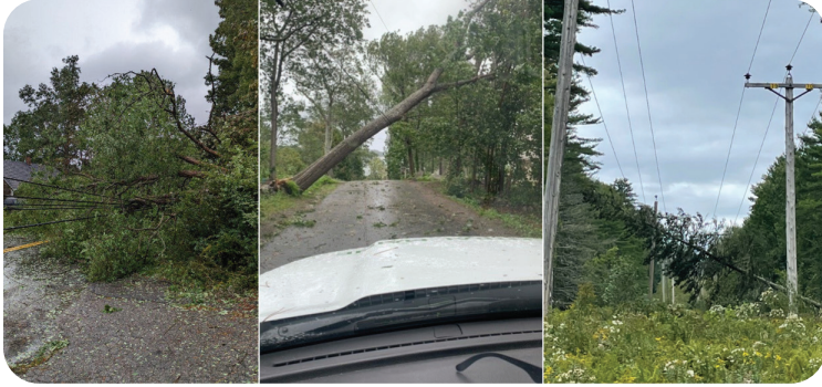
Damage from Hurricane Lee affecting more than 150,000 customers.
