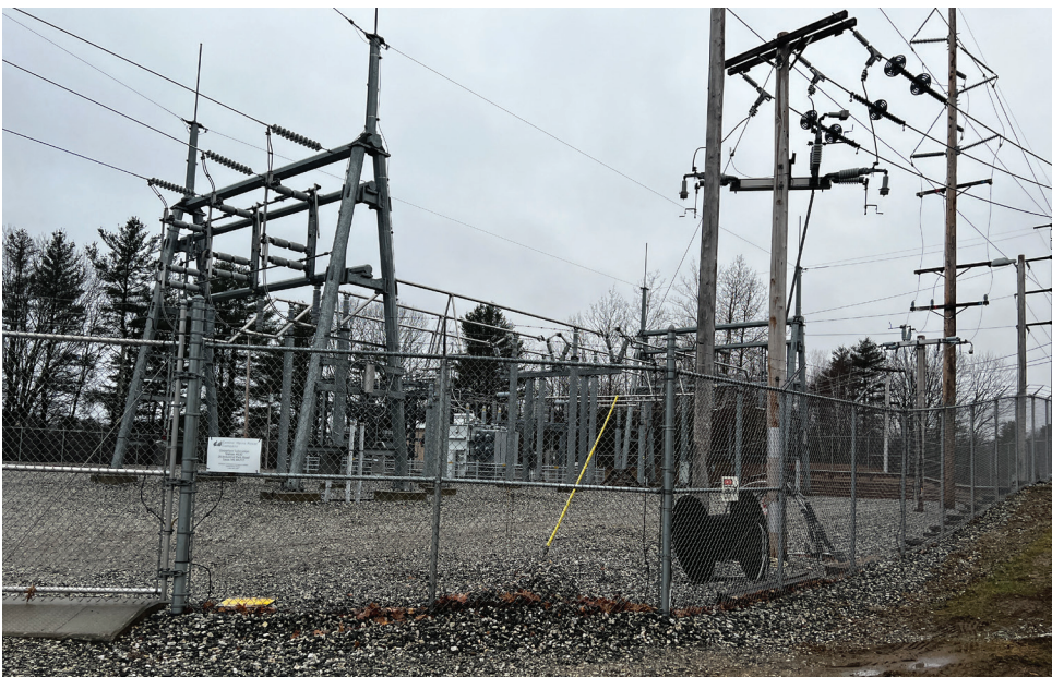
Goosefare Substation 26 Industrial Park Road Saco, Maine - April 2023.
