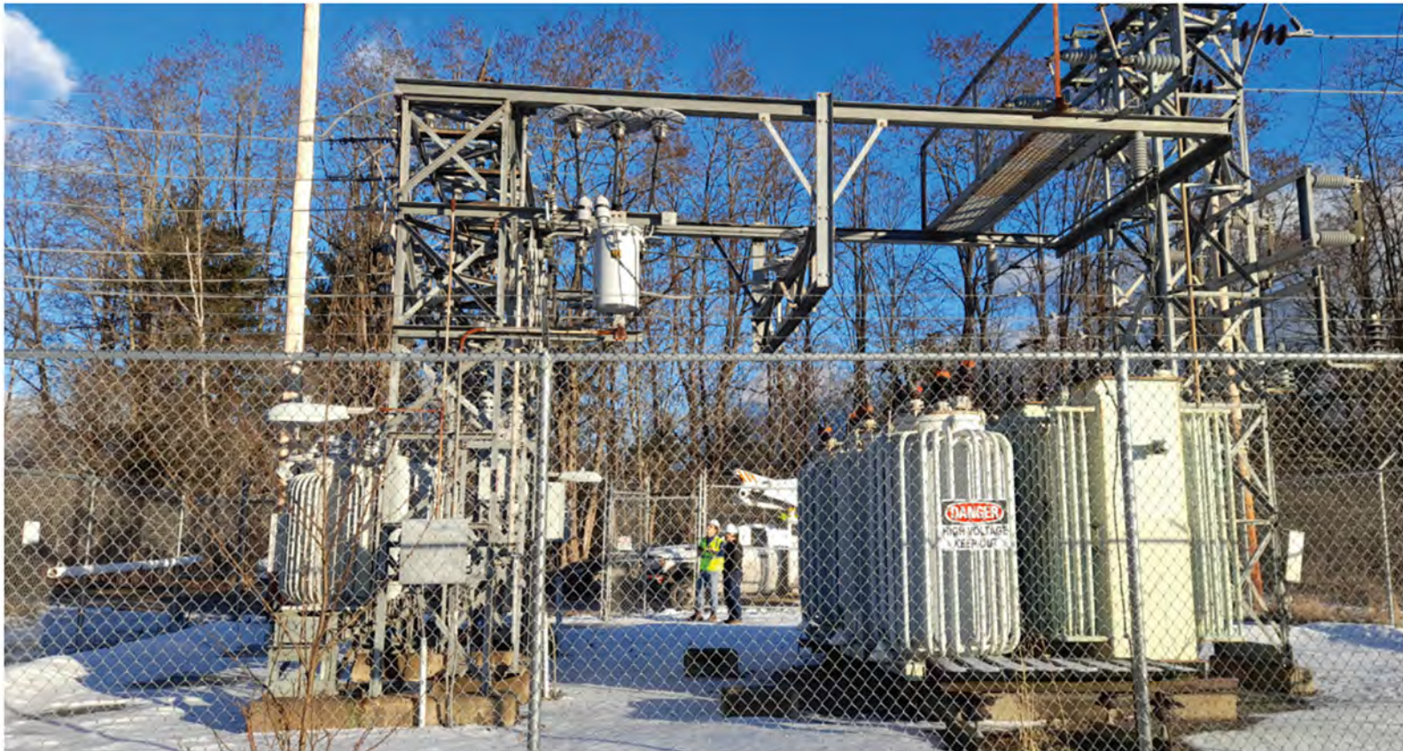
North Anson Substation, 905 River Road – December 2022
