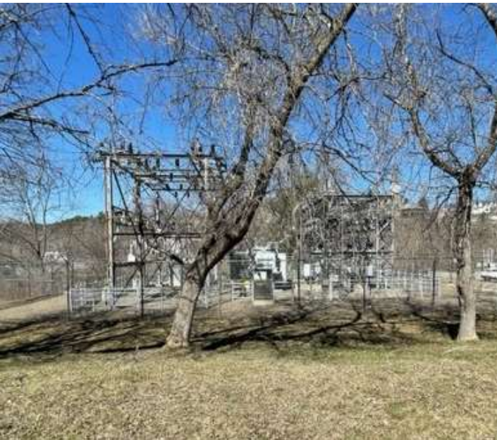
CMP's Bond Brook Substation is located on Mount Vernon Avenue in Augusta.
